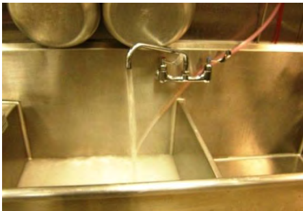
Figure 23. Filling of a 3-comp sink.
