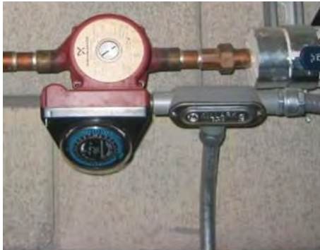
Figure 10. Timer mounted on a recirculation pump.
