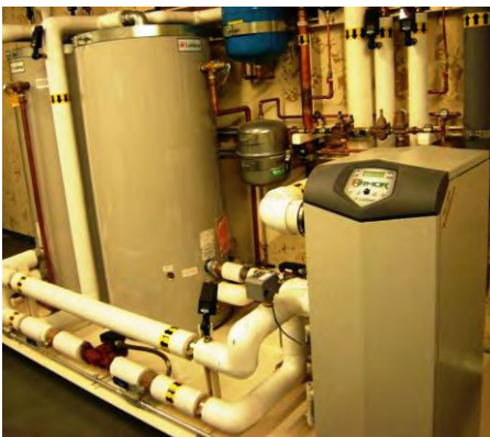
Figure 15. Water heating installations (a) storage water heaters (b) tankless units with controller, pump and storage tank (c) boiler with pump and storage tanks.
