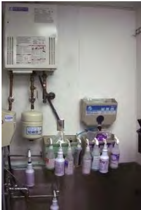
Figure 27. Tankless installed over mop sink.
