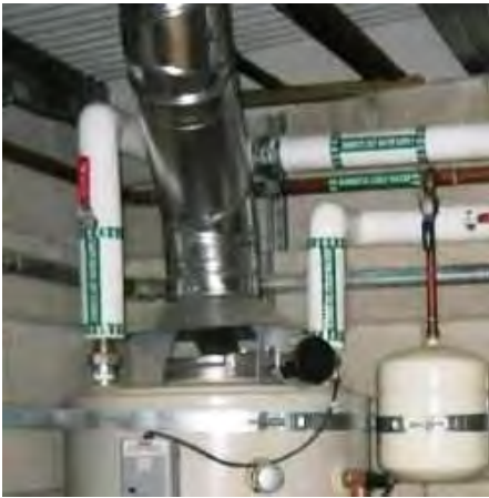
Figure 32. Stainless steel flue on storage heater.
