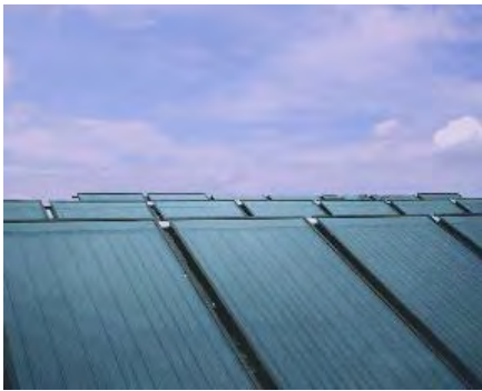
Figure 34. Solar thermal collectors.
