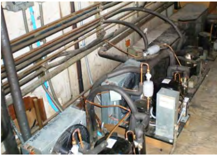
Figure 33. Refrigerant heat recovery tank and compressor/condenser unit.
